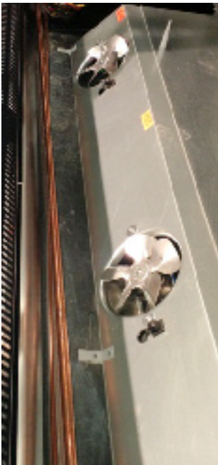
FIGURE 27: Fans and Case-to-Case Piping
