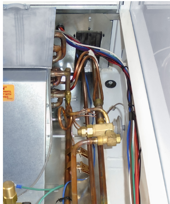
FIGURE 28: Expansion Valve Next to Evaporator Coil
