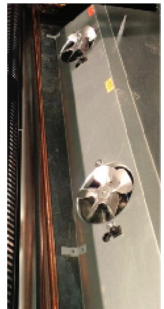
FIGURE 45: Fans and Case-to-Case Piping
